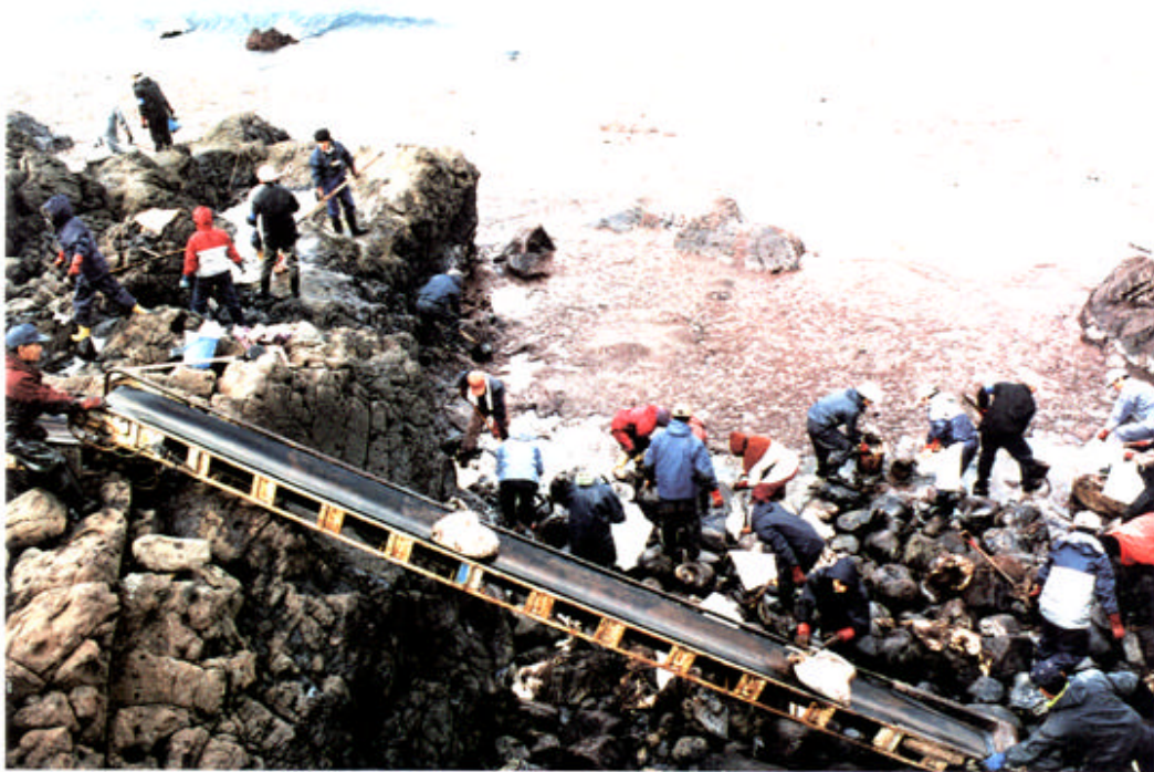
16 January Cleanup in rocky places with bad footing and dangerous conditions continues (Suzu City, Nagahashi Beach)
